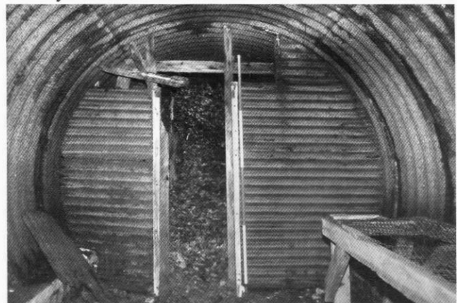
Arundel OB: the emergency exit, ventilation pipes and section of additional timber support frame
